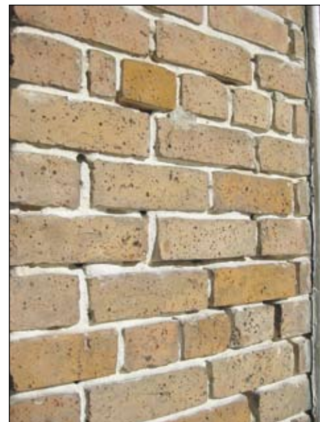
If your mortar looks like this: a powdery, sandy white substance, do not be alarmed. The mortar has simply reached the end of its life cycle. Hire a mason knowledgeable about historic brick, and he can restore your masonry structure in a process known as repointing.
