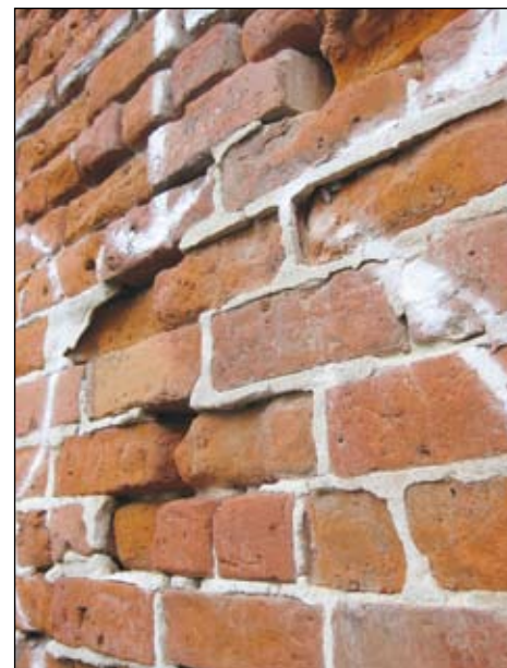
Portland cement mortar results in eroded and structurally unsound brick. These bricks have lost their strong outer face in a process known as spalling.
